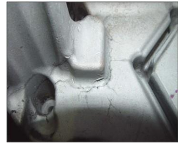
Figure 10 An example of gross crack.
